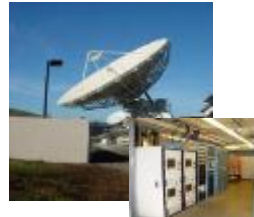
6 Ground Earth Stations
