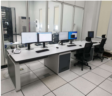
Engineering Support Room
